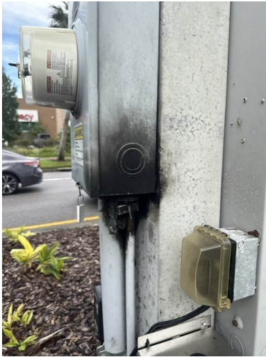
Electrical service equipment showing visible surge damage.
