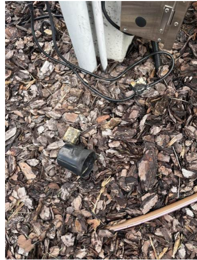
Dislodged surge-protection component near the lighting controls.
