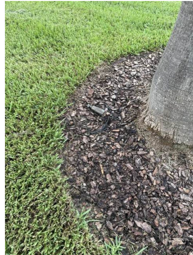
Displaced fixture and damaged mounting stake.
