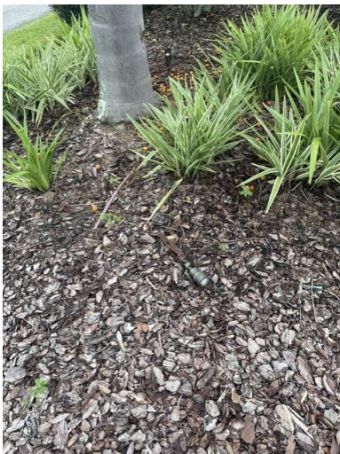
Fixture component separated from its installed position.
